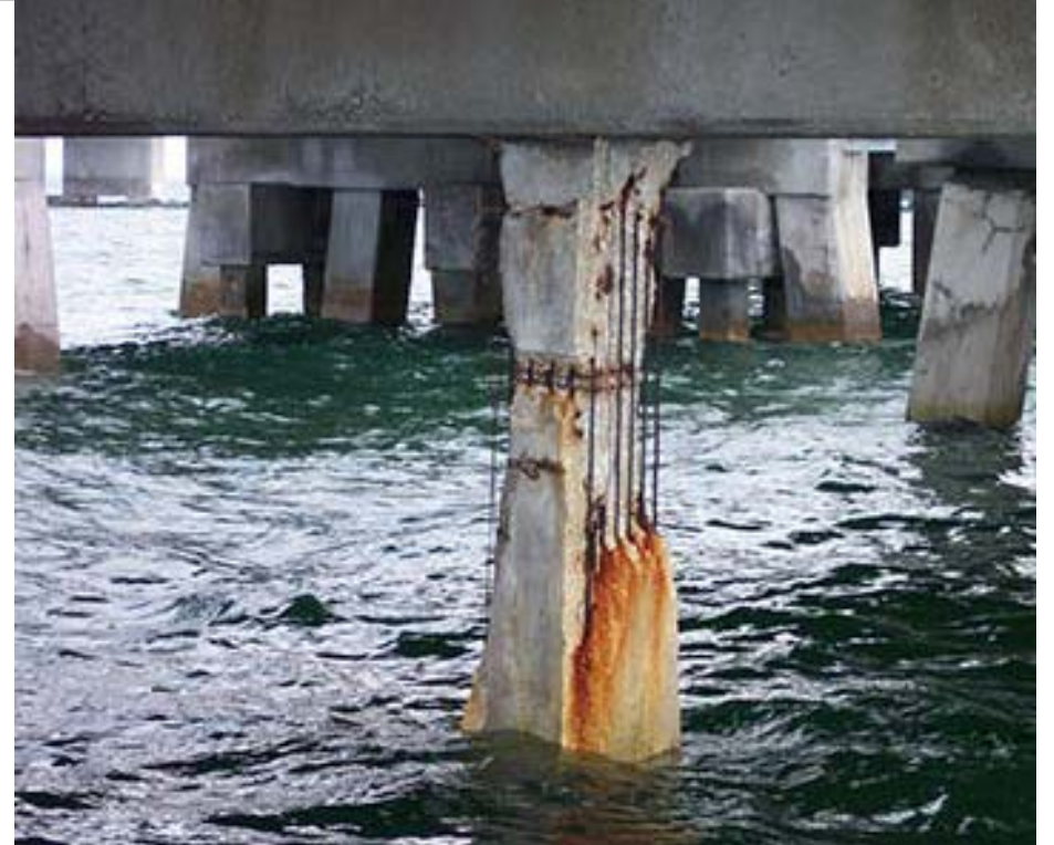
Bridge Piling with Damage Caused by Reinforcement Corrosion.
