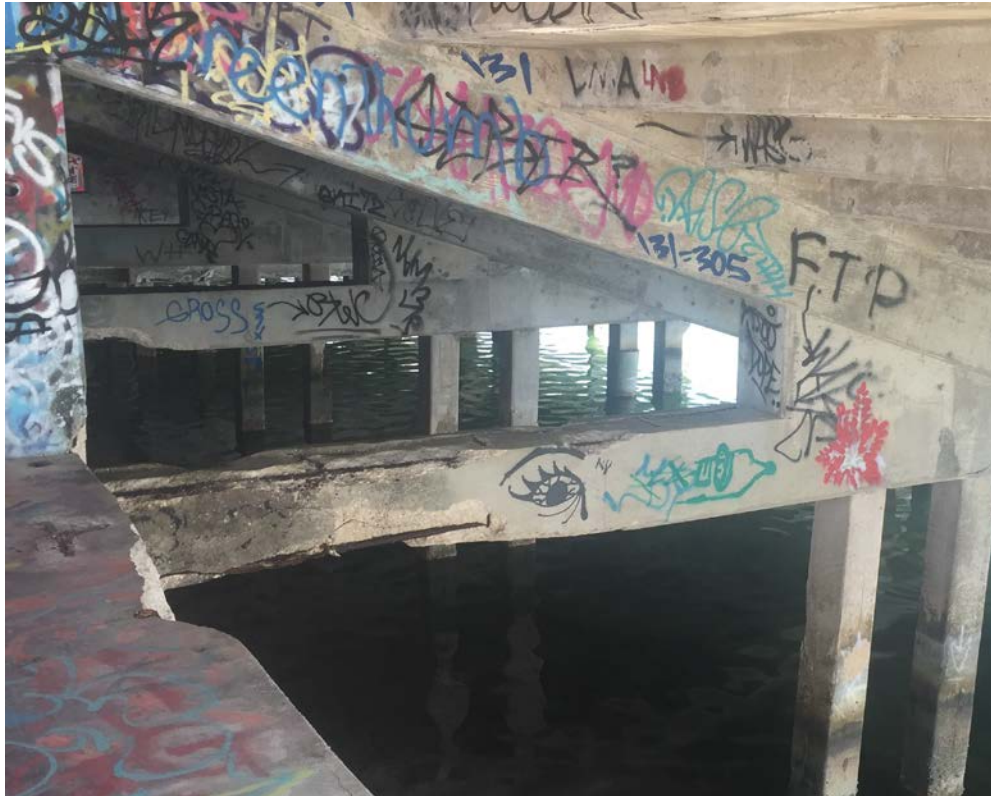
Miami Marine Stadium, beam with spall and corroded reinforcement.
