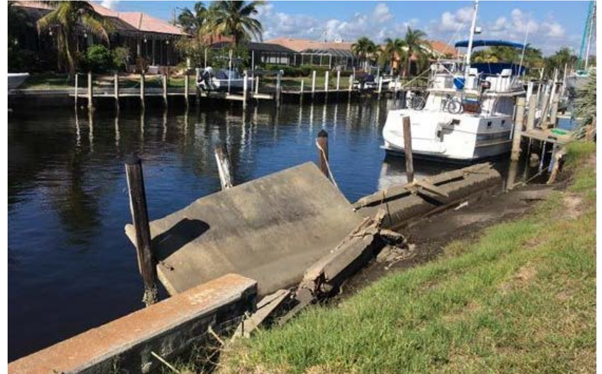
Collapsed Seawall due to Hurricane Irma in Punta Gorda, FL.
