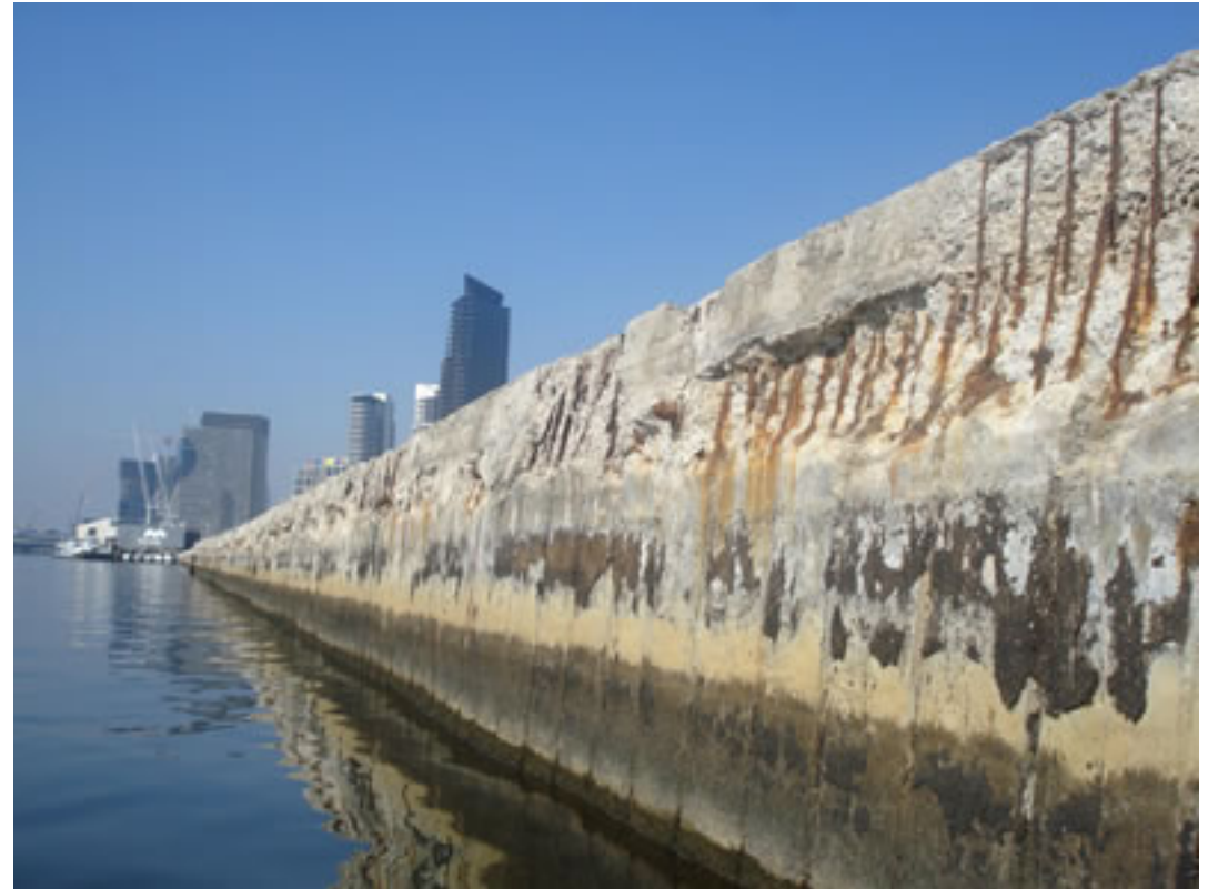
Bulkhead cap with reinforcement corrosion. Picture from Duoguard.
