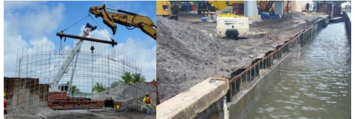
FDOT Bulkhead Rehabilitation Project. GFRP Used in Concrete Cap and Fascia Panels
